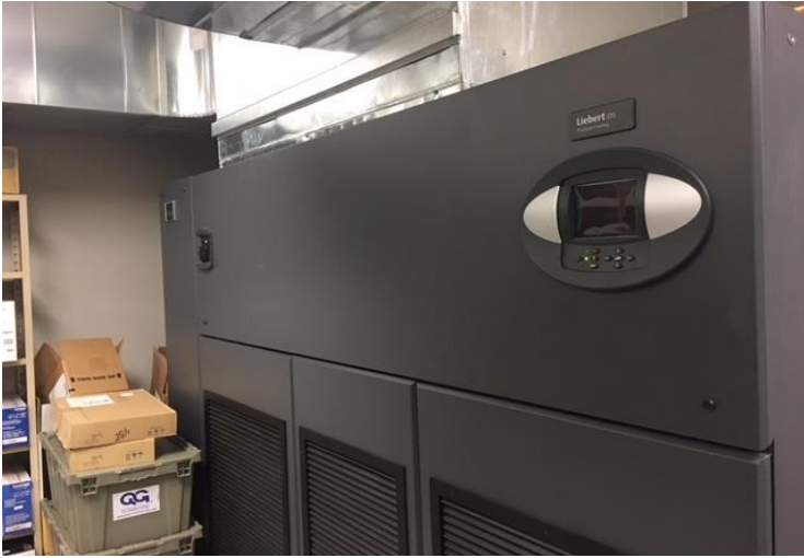
LIEBERT HVAC 12.5 TON COLLING SYSTEMS
